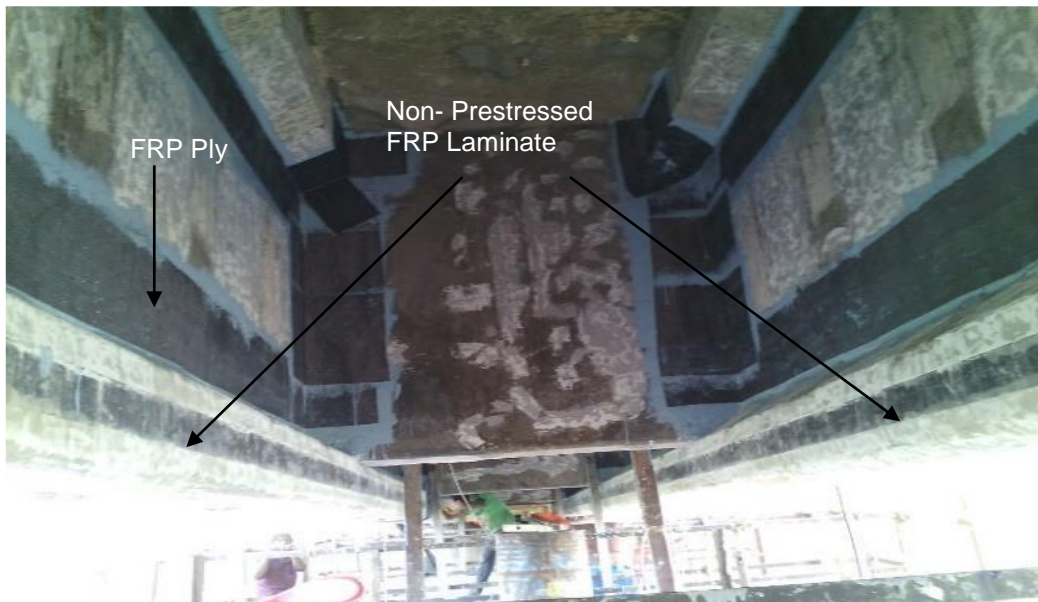
Figure 9. FRP ply and Non-Prestressed laminate applied to inner face side of PSC I girder
