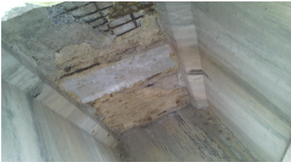
Figure 1. Cover delamination and corroded reinforcement exposure observed in deck slab bottom
