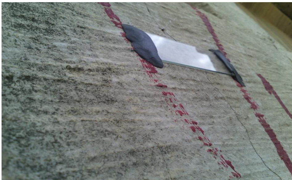
Figure 2. Severe cracks seen in girder
